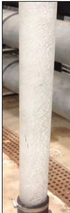
Figure 39: Close-Up of Air in Perspex Pipe. System On.
